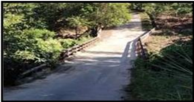
Fig. 16: Narrow Bridge without Pedestrian facilities (Road #6)
