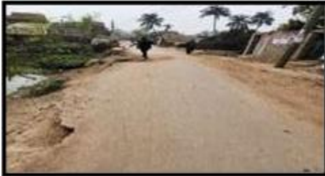
Fig. 7: Traffic Movement Hamper Due to Lack of Maintenance Work (Road # 5)
