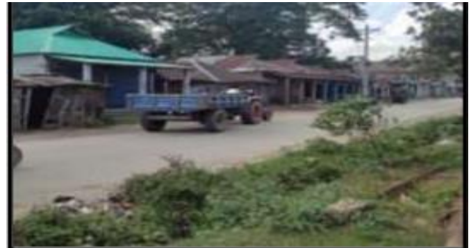
Fig. 12: Roadside Open Drain Without Barriers (Road # 02)
